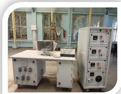
Circuit Breaker Analyzer
