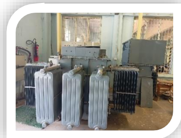
1-Ø 10000 A (AC) Transformer
