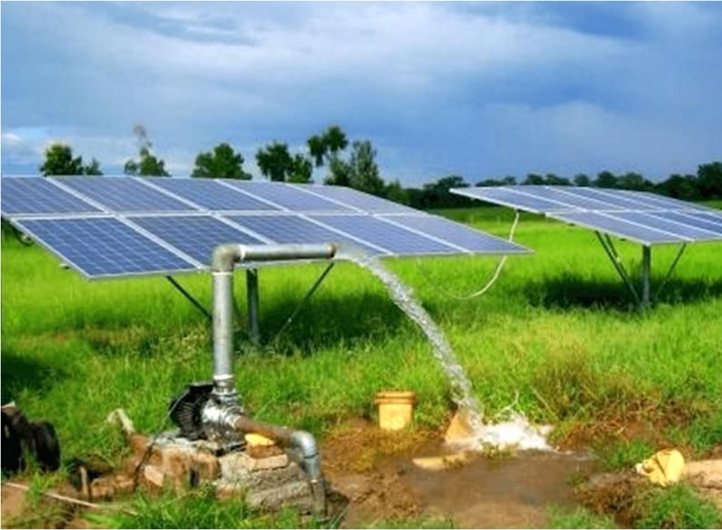
Photovoltaic Solar Water Pumping System.
